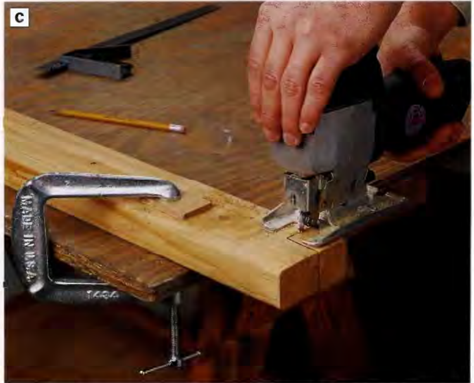
PHOTO C: Notch the top front corner of the center front leg so it will fit around the top front stretcher. Then combine this leg with the rear support, drawer stretcher, drawer slide and lower stretcher to form the middle support assembly.
