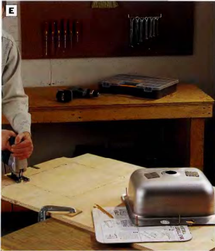
PHOTO E: Center the sink so it will hang over the storage area on the left side of the bench. Lay out the sink opening using the template provided by the manufacturer, and cut out the sink opening.
