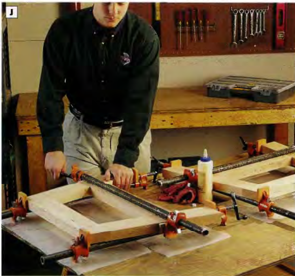
PHOTO J: Build the glider stand ends by attaching the top and bottom end rails to the stand legs with dowels and glue. The bottom rails fit between the legs, while the top rails overlap the top ends of the legs.
