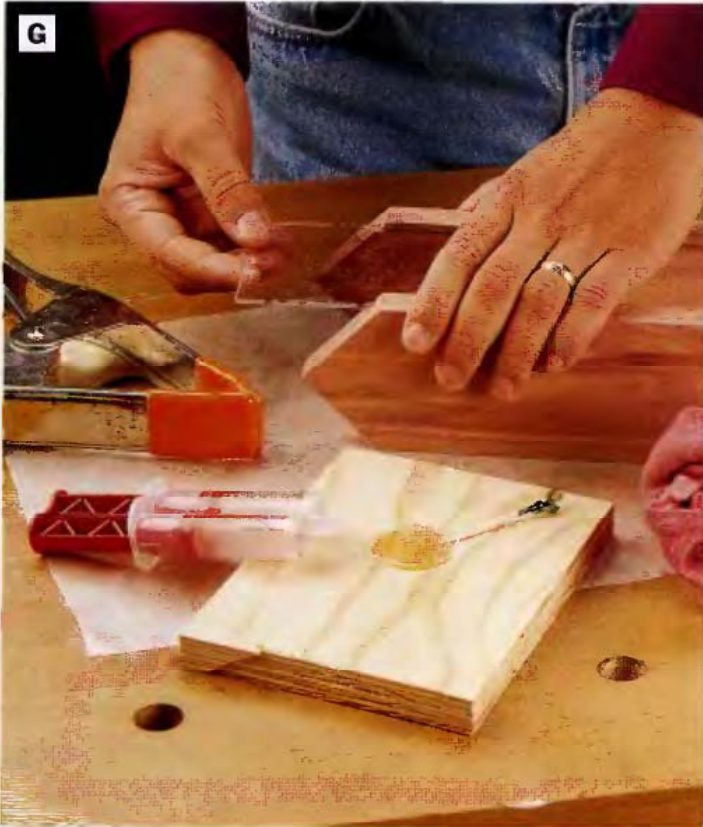
PHOTO G: Spread two-part epoxy into the grooves in the side panels, remove the protective film from the Plexiglas end pieces, and slide the end pieces into the grooves. The end pieces should stop \frac{3}{4} in. from the bottoms of the sides.
