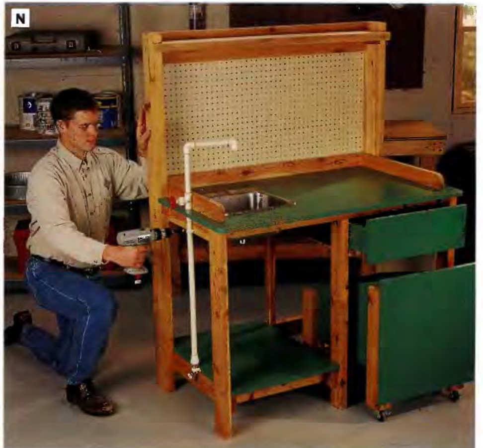
PHOTO N: Use strap clamps to attach the plumbing assembly to the bench.
