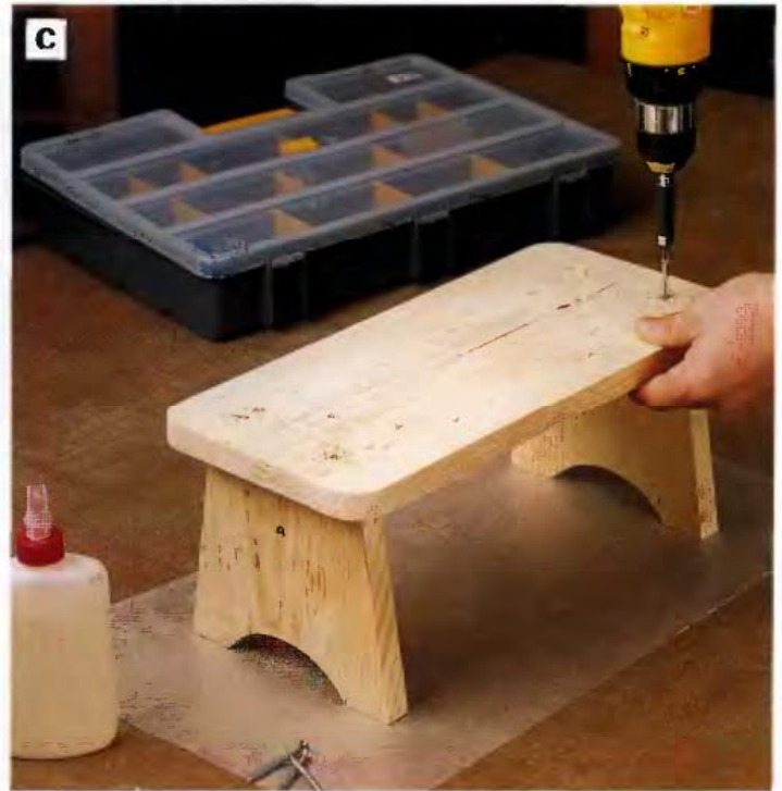
PHOTO C: Attach the top to the stretcher and legs with glue and screws. Lay out the stretcher and leg locations on the top first, for locating the screws.
