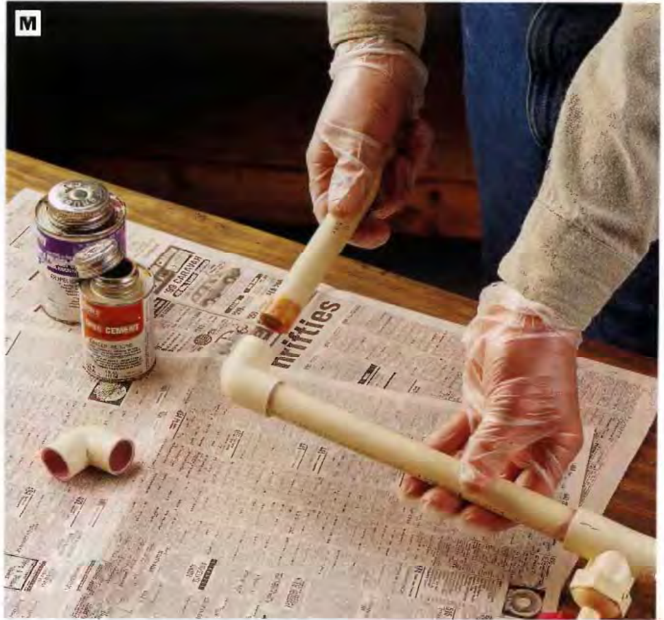
PHOTO M: Cut the straight pipe sections to length and dry-assemble the entire plumbing unit to check its fit on the potting bench. Then disassemble the PVC, prime the mating parts of each joint, and bond the PVC together with CPVC cement. Wear gloves when bonding the parts.
