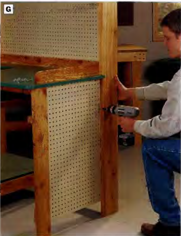
PHOTO G: Fasten the perfbboard side and back panels to the bench framework with 1½-in. galvanized deck screws. Be careful not to overdrive the screws when installing the perfbboard.
